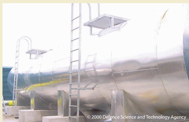
An ice-storage tank in use at Changi Naval Base.
